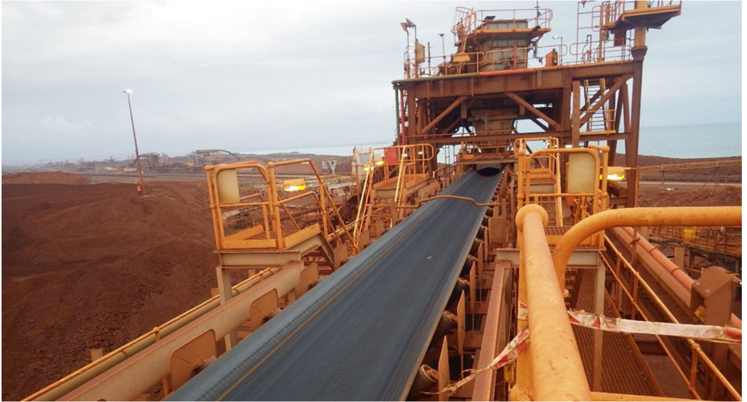
Major iron ore port loading facility in the Pilbara Western Australia
